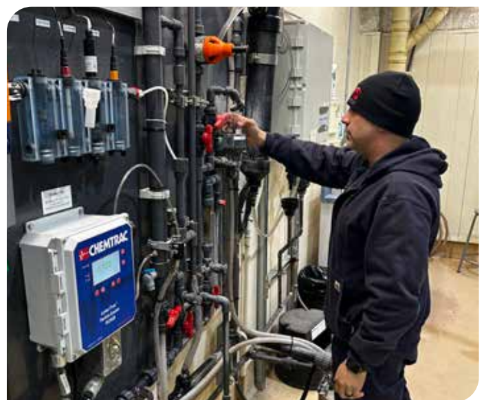
WTP Lead Electrician Cosimo Crupi verifying instrument readings at the raw water - water quality station at the Bare Point WTP
