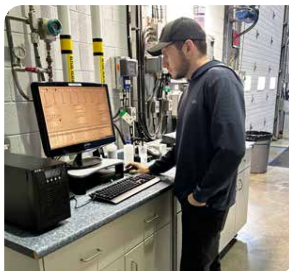
WTP Operator Thomas Parkin monitoring SCADA at the final water - water quality station at the Bare Point WTP
